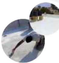
Cool Roof Paints
