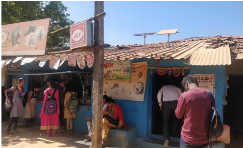
Before: Due to standard construction techniques of tin sheet roofing, low ceiling and lack of openings like windows
