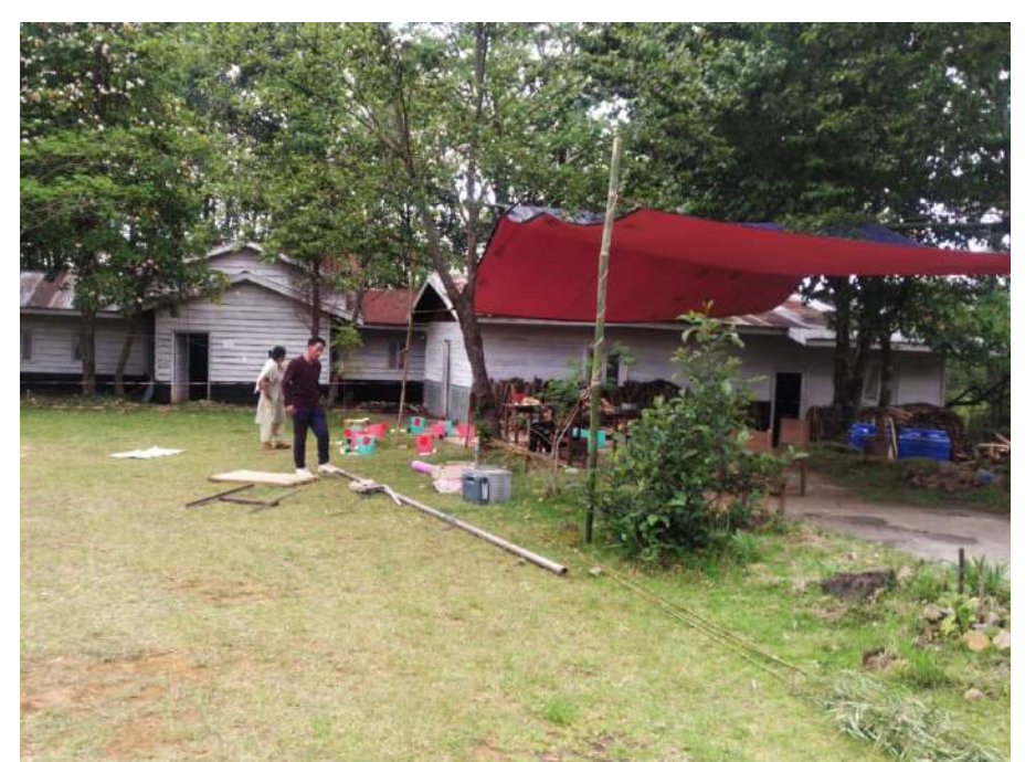
Pictures: Team of SNL installing solar energy systems for Quarantine Centres, established by Volunteers for Village Development (VVD) Training Centres in Ukhrul District, Manipur
