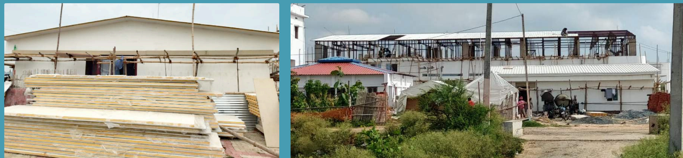
Ongoing construction at the Vistex Hospital in Bihar using Pre-Fab and Pre-Cast Materials
