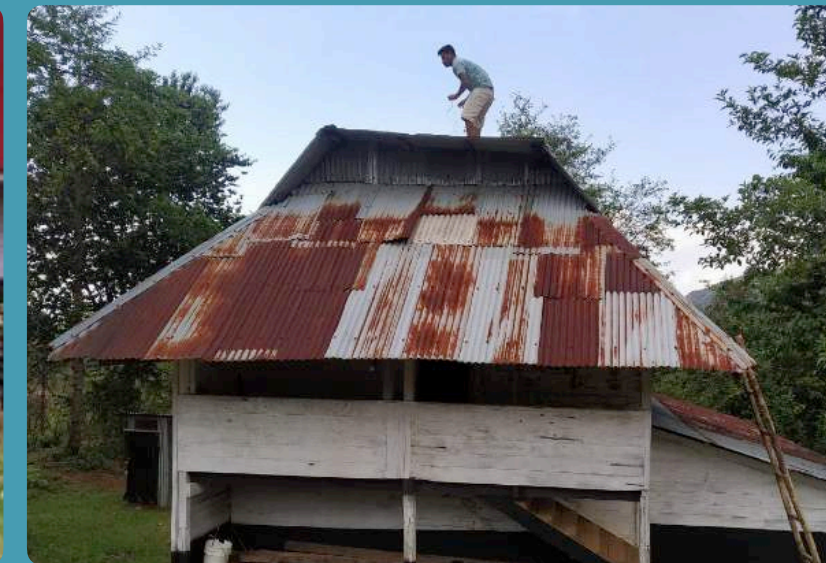
Volunteers for Village Development (VVD) Training Centres identified for Quarantine in Ukhrul District, Manipur- Installation in progress across identified quarantine centres
