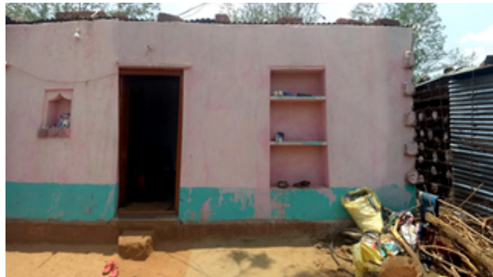
BEFORE: Indoor Temperature was recorded 6°C higher than outdoor temperature
